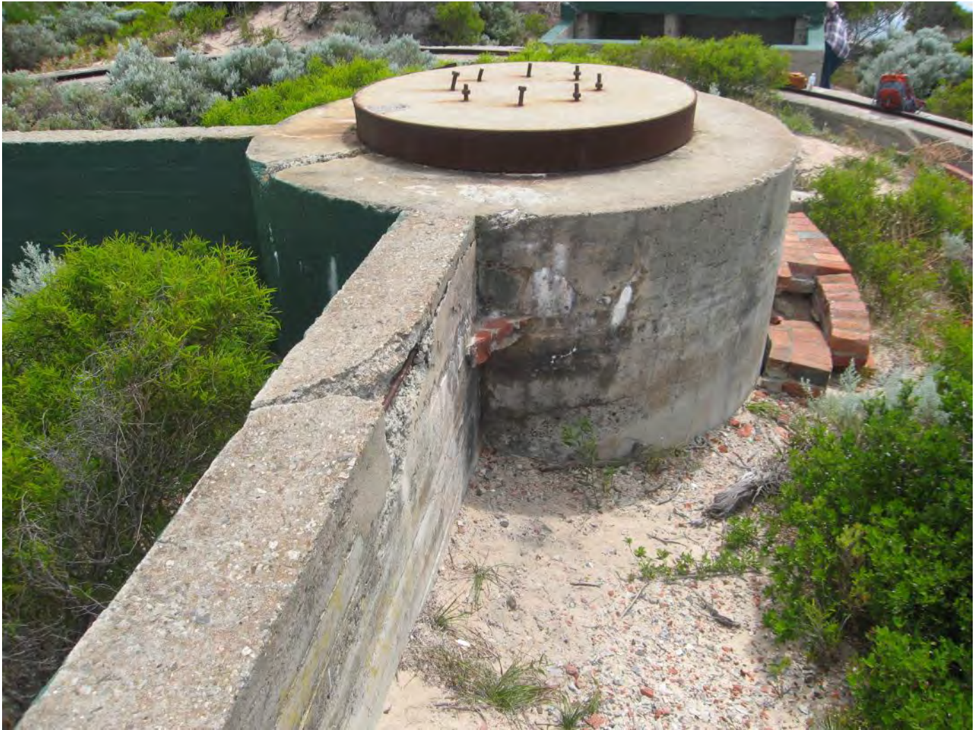
Figure 101: Gun Emplacement - rusted steel reinforcements causing chunks of concrete to blow and break off
