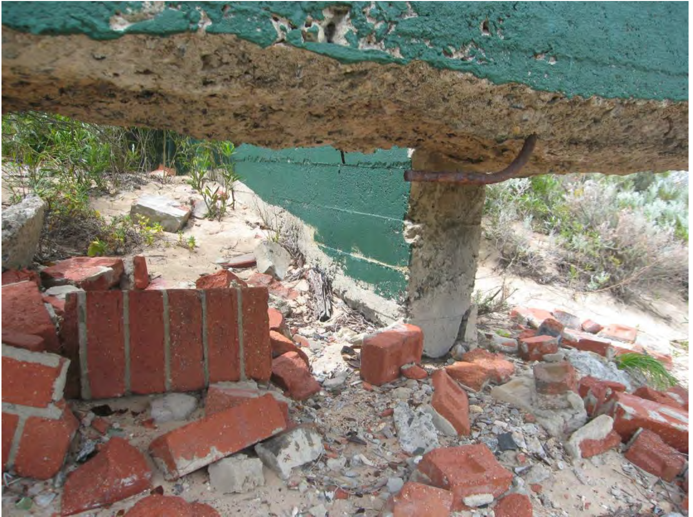
Figure 104: Gun Emplacement - underside of the concrete structure
