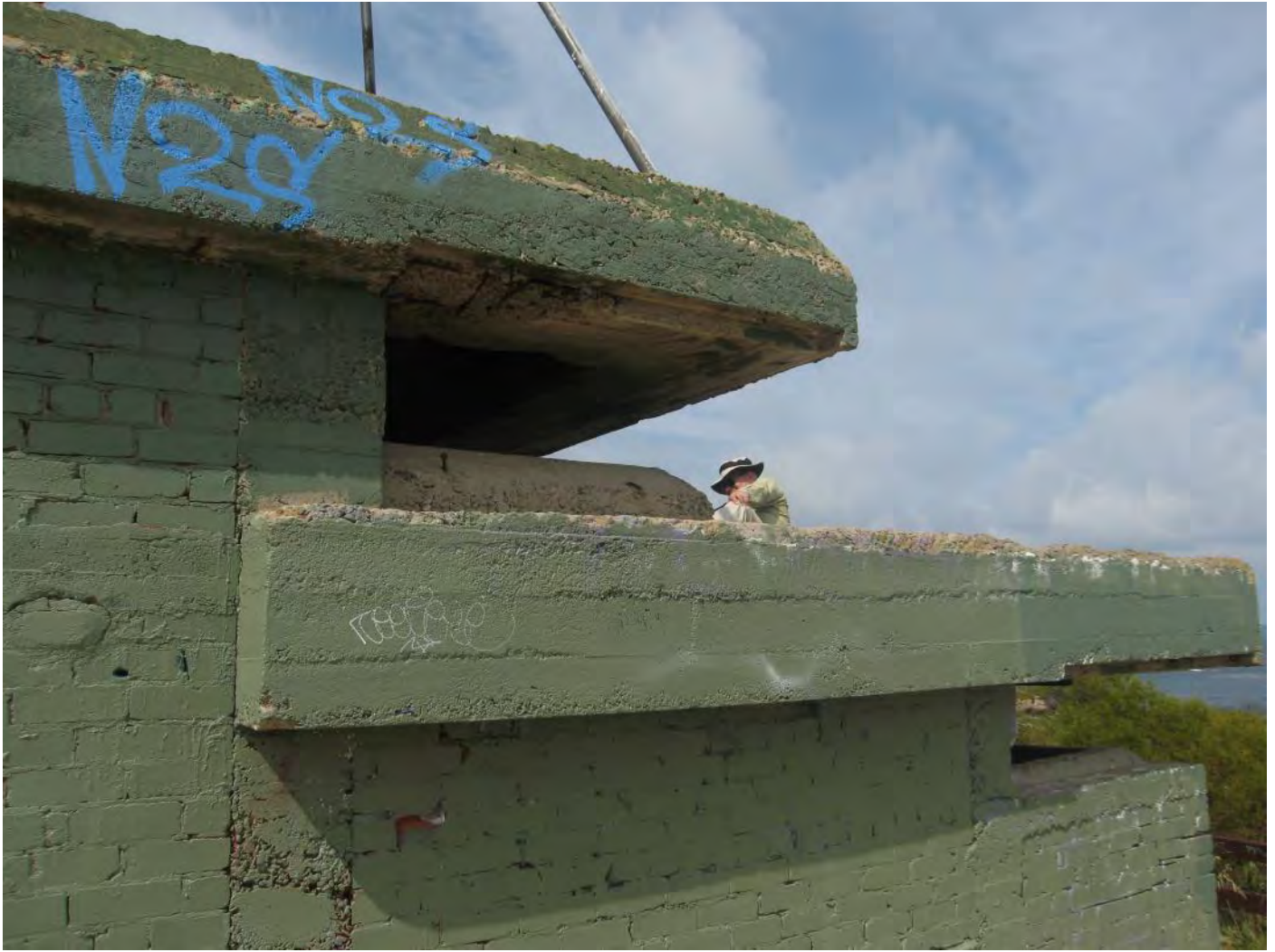
Figure 65: North Elevation – concrete overhang to the roofs providing protection to the observation openings
