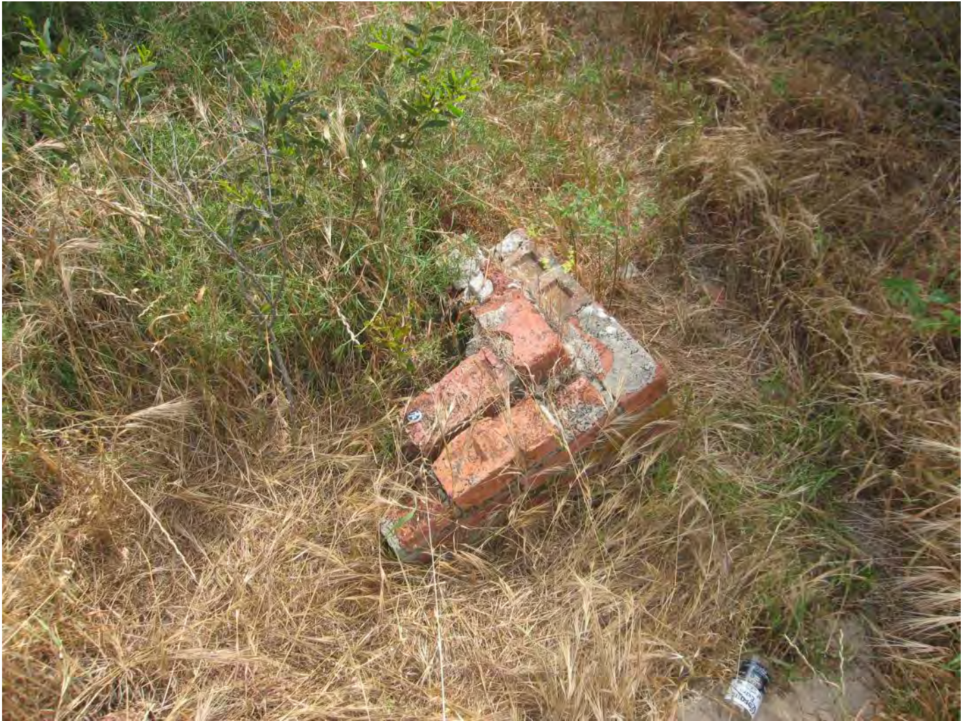
Figure 87: Operations Bunker – Remnant fabric lying close by the east elevation of the structure
