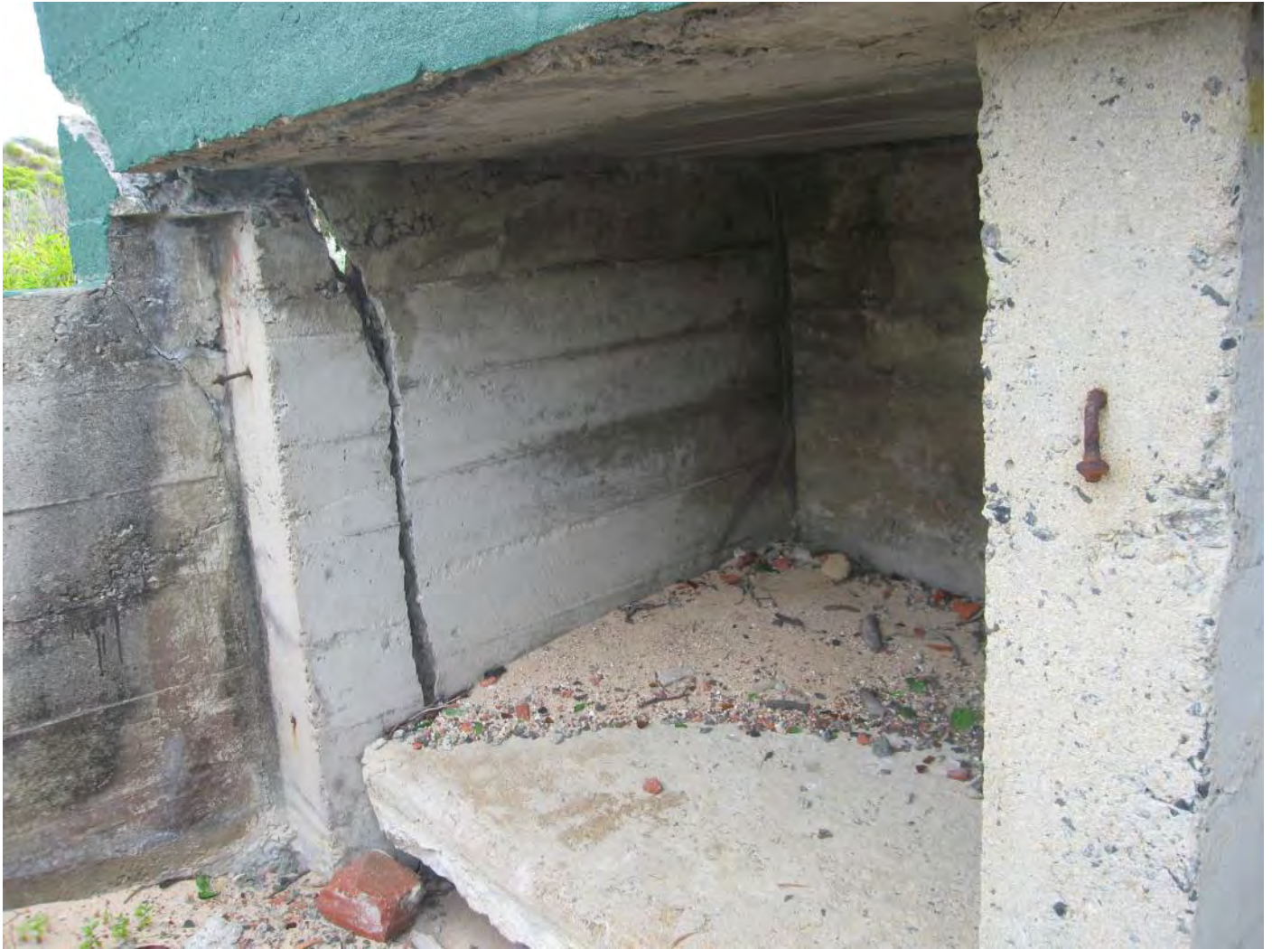
Figure 110: Gun Emplacement - Cracking in the framework of Ammunition Store No. 1
