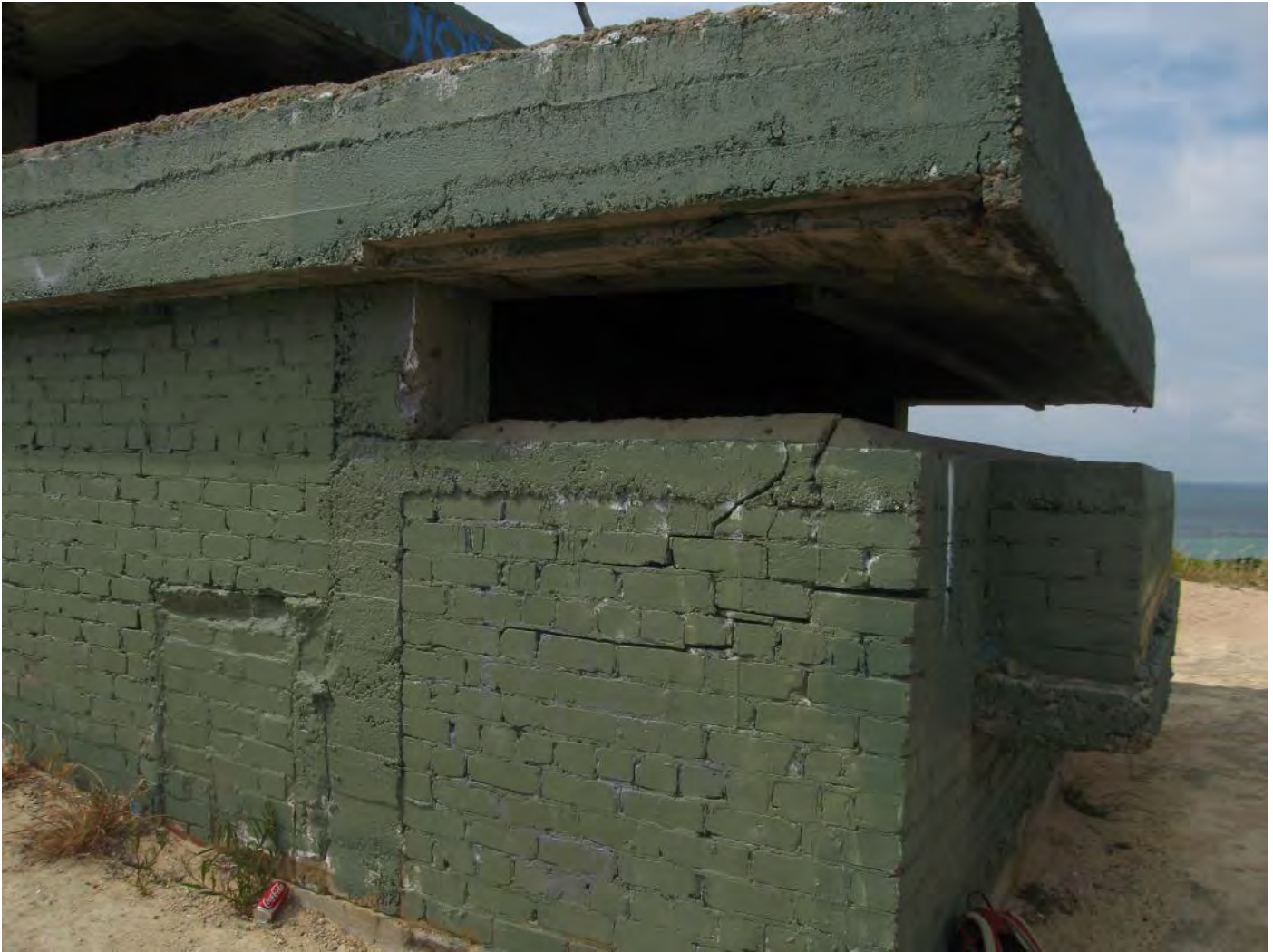
Figure 63: North Elevation – western corner being pulled away from the main elevation
