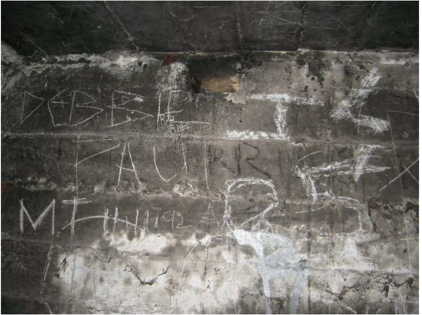
Figure 123: Ammunition Bunker – graffiti in Room 1
