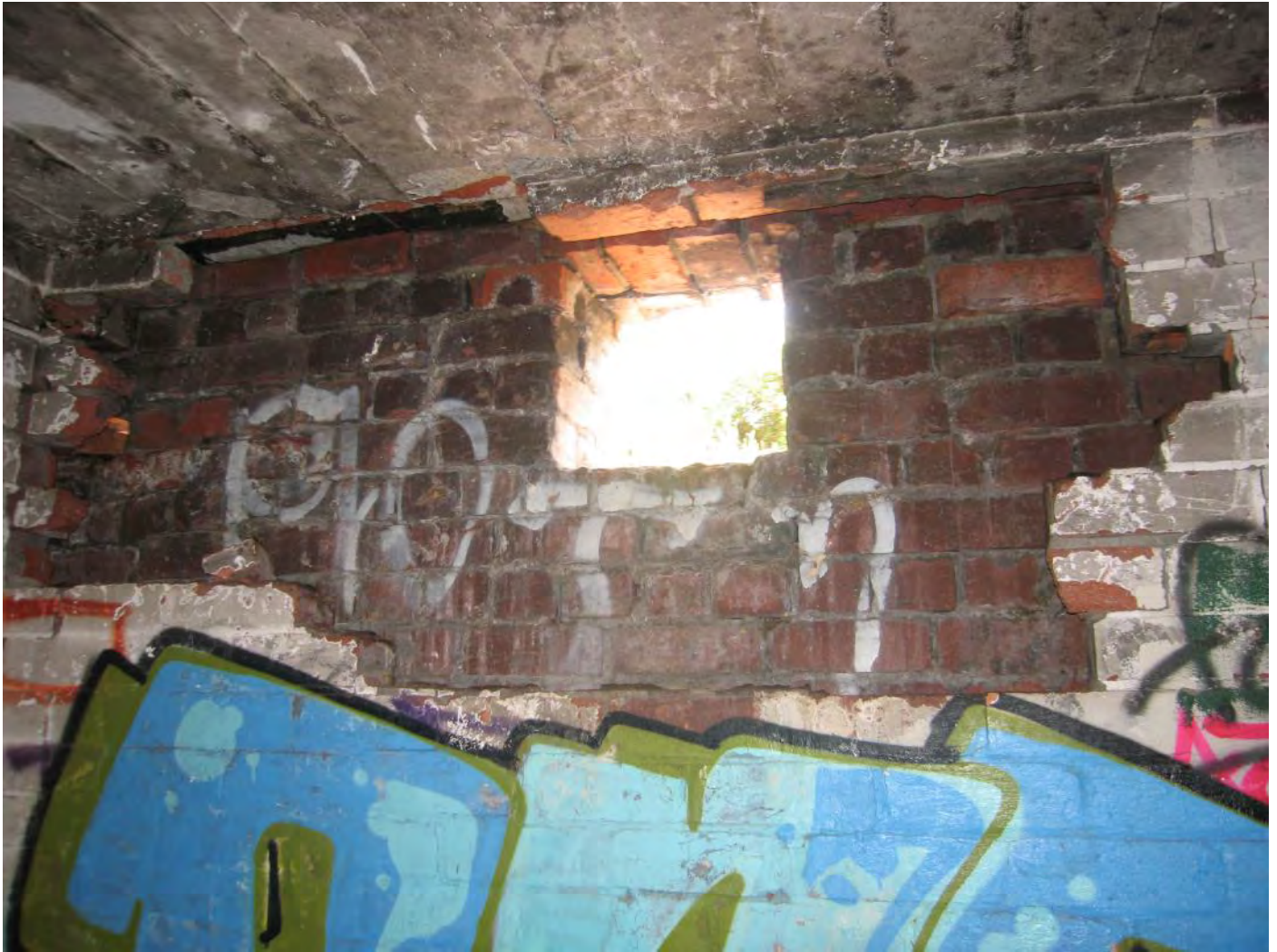
Figure 94: Operations Bunker – Small opening in north wall with damaged brickwork
