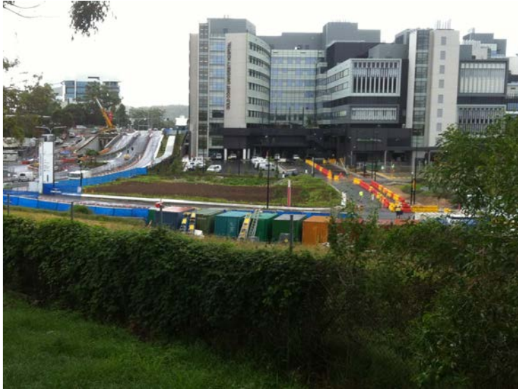
The 750 bed GCUH is almost complete, with the underground light rail station under construction to the left
