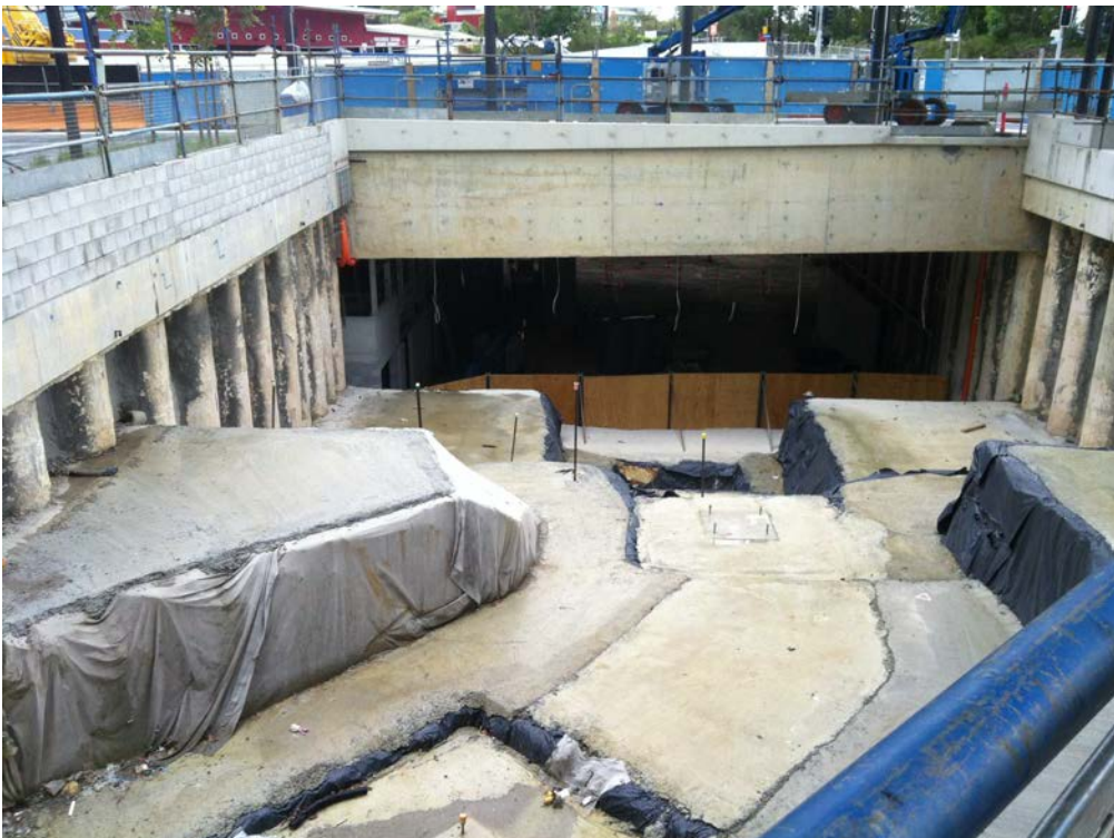
The underground light rail station is the most northern stop for Stage 1 of the Gold Coast Rapid Transit project
