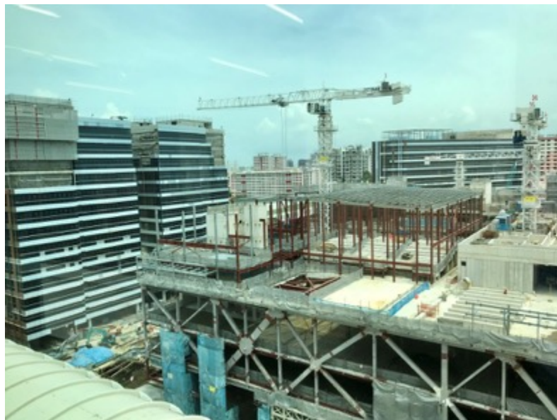
The viewing area of the Paya Lebar Quarter development site from inside Lendlease's office (below)
