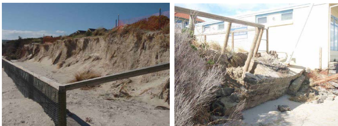
The Carrum foreshore is subject to erosion from storm surges and rising sea levels
