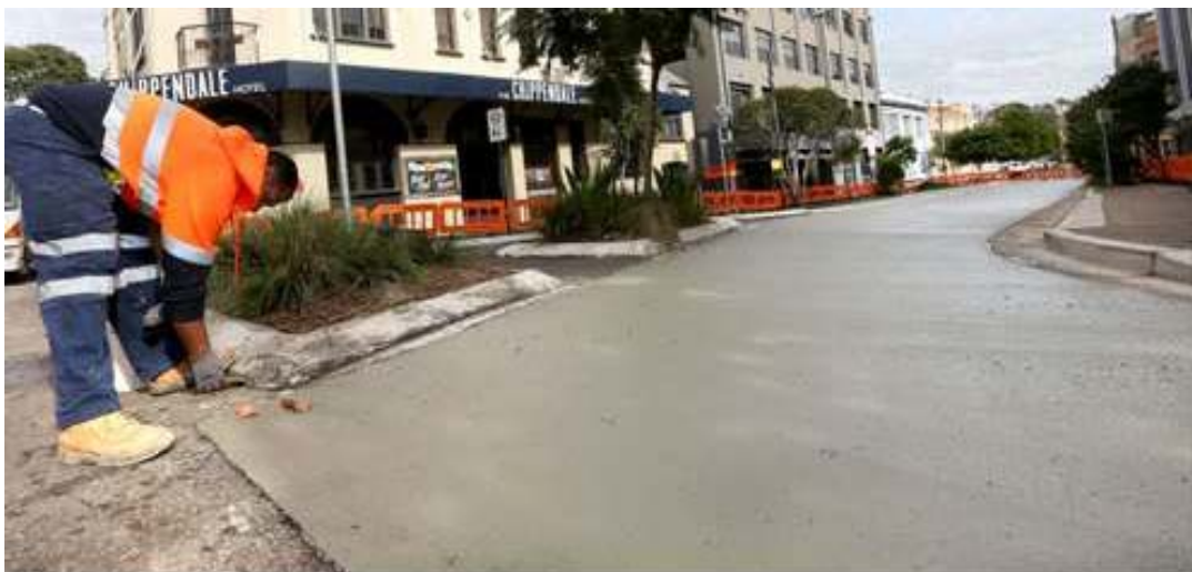
Although of limited success, the light road pavement trial provided the City of Sydney will useful information to apply to other areas.
