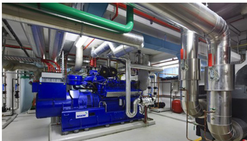
Tri-generation Energy Plant
