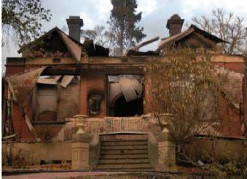
Fire damage caused by local bushfire
