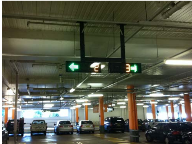
The car parks beneath the town centre include signage with directional arrows showing availability of empty car parking bays
