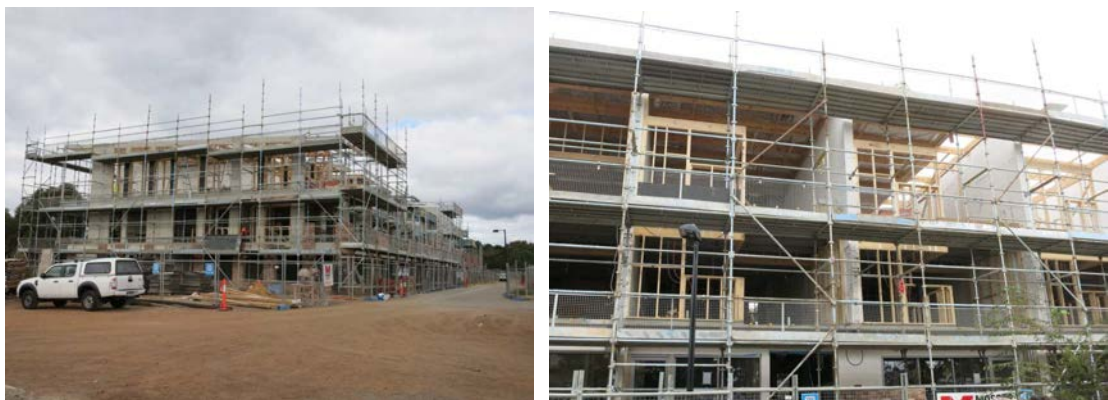
The housing mix currently under construction at Bowden includes 3-4 story townhouses and apartments
