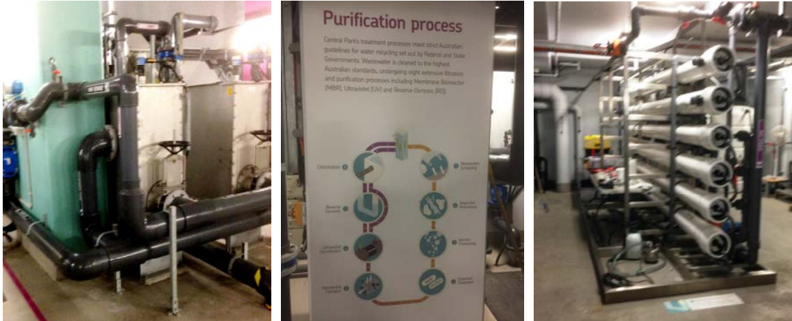
The wastewater treatment plant produces recycled water for non-potable uses throughout the development, with recycled/treated stormwater harvested for landscaping and green wall irrigation
