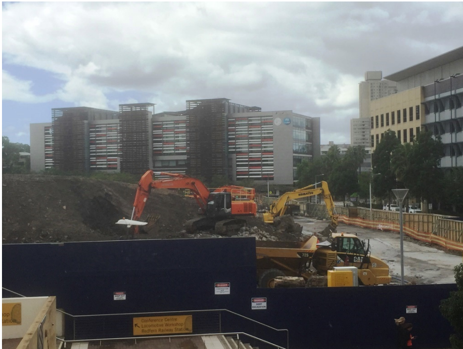
One of the CBA office buildings under construction at the ATP site
